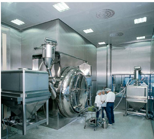
Pharmaceutical cleanroom with Viledon HEPA filters
