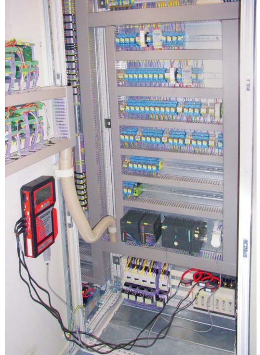
Control cabinet with an eTracker measuring instrument connected up
