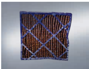
Pleated Filter with moisture damage and microbial growth
