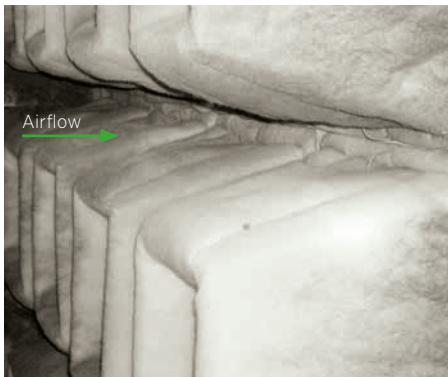
The TRI-CUBE RFX filters installed
